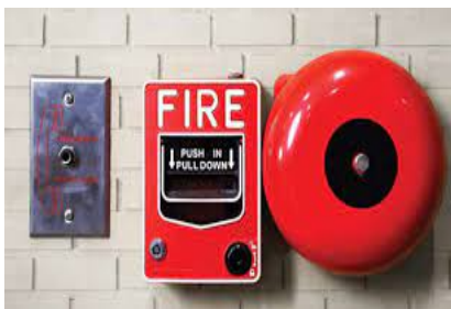
FIRE ALARM AND SAFETY
